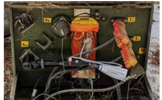
Figure 2: MIC Injection in a low-profile transformer
