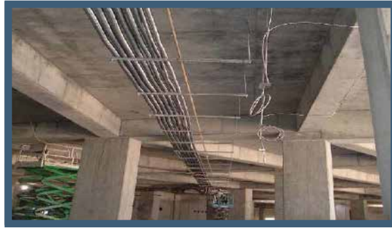
MC cable using trapeze support system
