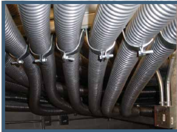
MC cable secured every 6' with straps and clamp
