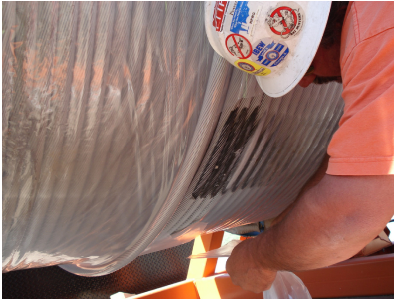
Figure 4. Water stain on conductor.
