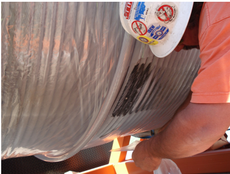
Figure 5. Water stain on conductor.
