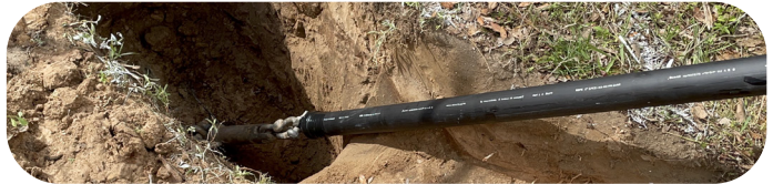
The CIC, gripped by a pulling eye, is unwound from the reel and is pulled underground through a small pilot hole pre-made by the HDD drill bit.
