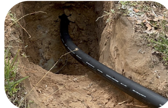
200 feet of CIC is continuously pulled by the HDD equipment into a small channel. This narrow pathway was pre-drilled by the bore to accommodate the specific size of the CIC pipe.
