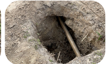
The full length of CIC has been pulled all the way to the end point where the HDD pulling equipment is located. This concluded the install of the new below-grade circuit for one residential segment.
