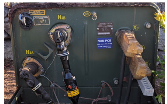
Figure 2: MIC termination in a transformer.
